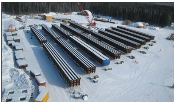
Left: Aerial photos taken by ARRC Board Director John Binkley in late March 2013 show bridge construction activity. Top: progress made on the bridge pier foundations. Bottom: Girders are bolted together into spans in the construction yard. Spans will eventually be set upon the piers.
